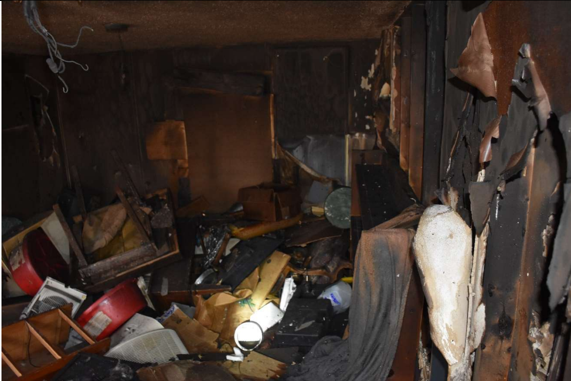
Figure 5 Photograph NJF_0024, Open area with smoke staining and charring to wall paper.
