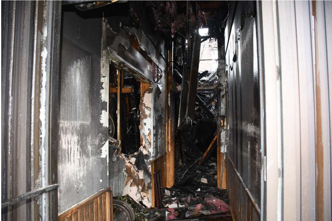
Figure 6 DSC_0076.JPG Interior of South Hallway, Collapse, Soot Deposits
