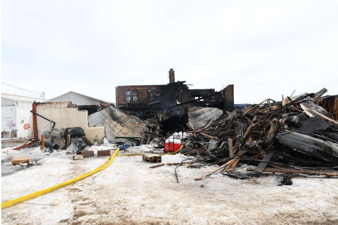
Figure 3 Photograph DSC_0013.JPG Exterior East Wall, Collapse, Gas Meter
