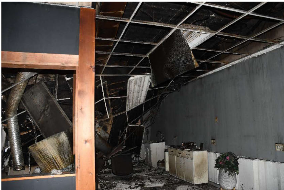
Figure 10 Photograph DSC_0019.JPG Interior of Northeast Business, Interior West Area, North Wall, Ceiling Collapse
